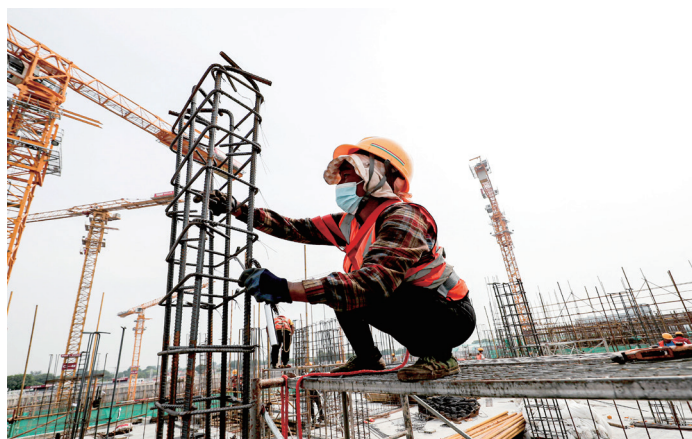
A worker binds steel bars at a construction site to build placement housing for residents in Tongzhou District, Beijing, which is a key project the district implements to improve people's wellbeing. Photo: CFP
